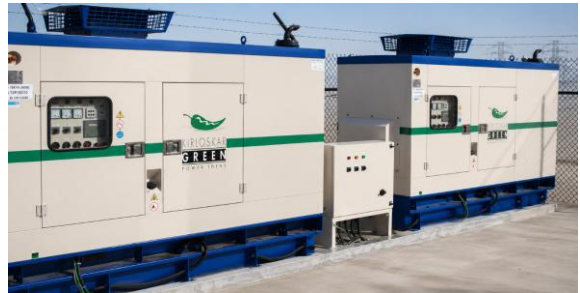
STC Network, KSA
