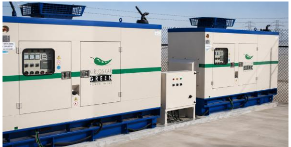
STC Network, KSA
