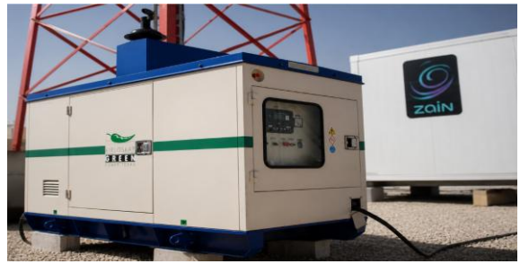
ZAIN Telecom, KSA
