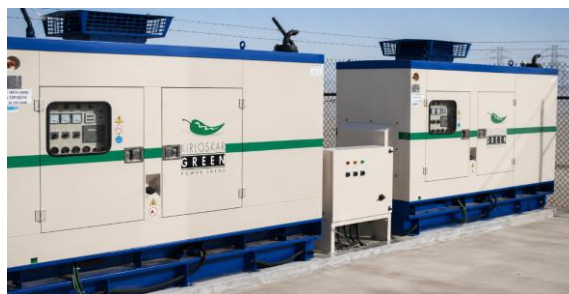
STC Network, KSA
